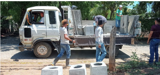
Delivery of the concrete bases and seats for the latrines. Installation is by workers skilled in masonry & metal fabrication.
