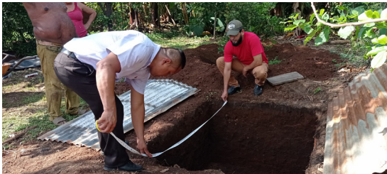
Beneficiaries aid in the construction of latrines, a process which is closely monitored to insure they meet minimum standards
